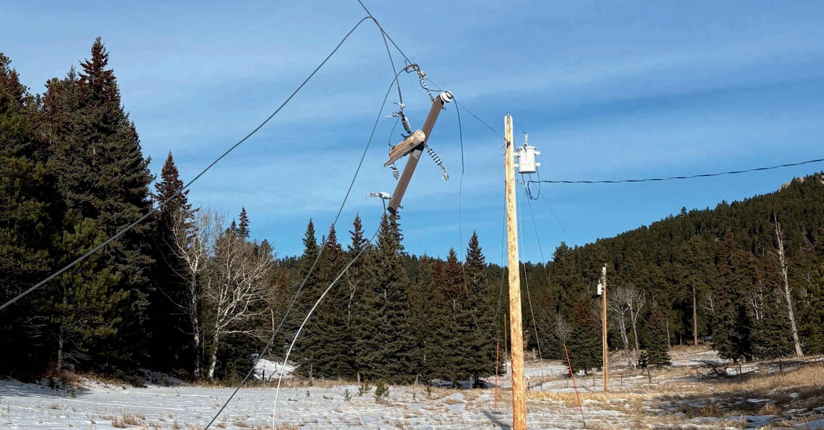
Intense wind left the crossarm of a broken three-phase pole hanging after a holiday storm. Photos submitted by Black Hills Electric Cooperative
